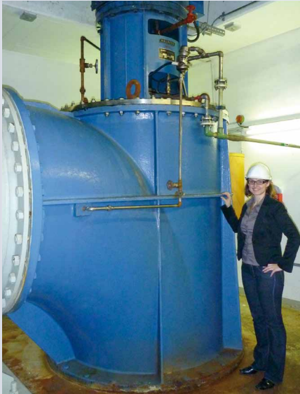
Main cooling water in the Rostock power station
